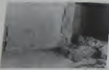
FIG. 25. A. N. S. Nino. Left-hand shoulder of doorway of masonry which was subsequently sealed up.
